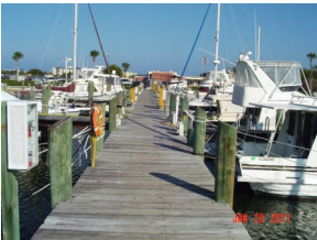
NB Dock prior to re-decking
